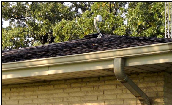
Typical HCN Rooftop Antenna Installation
